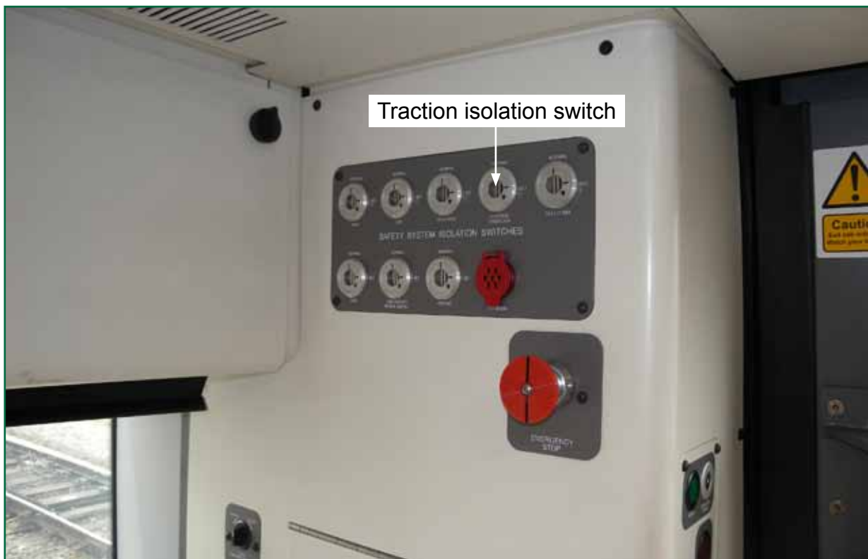
Figure 11: Traction Isolation Switch (TIS)
