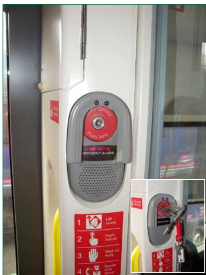
Figure 8: Passenger communication alarm with alarm active (inset - alarm being manually reset using a key)
