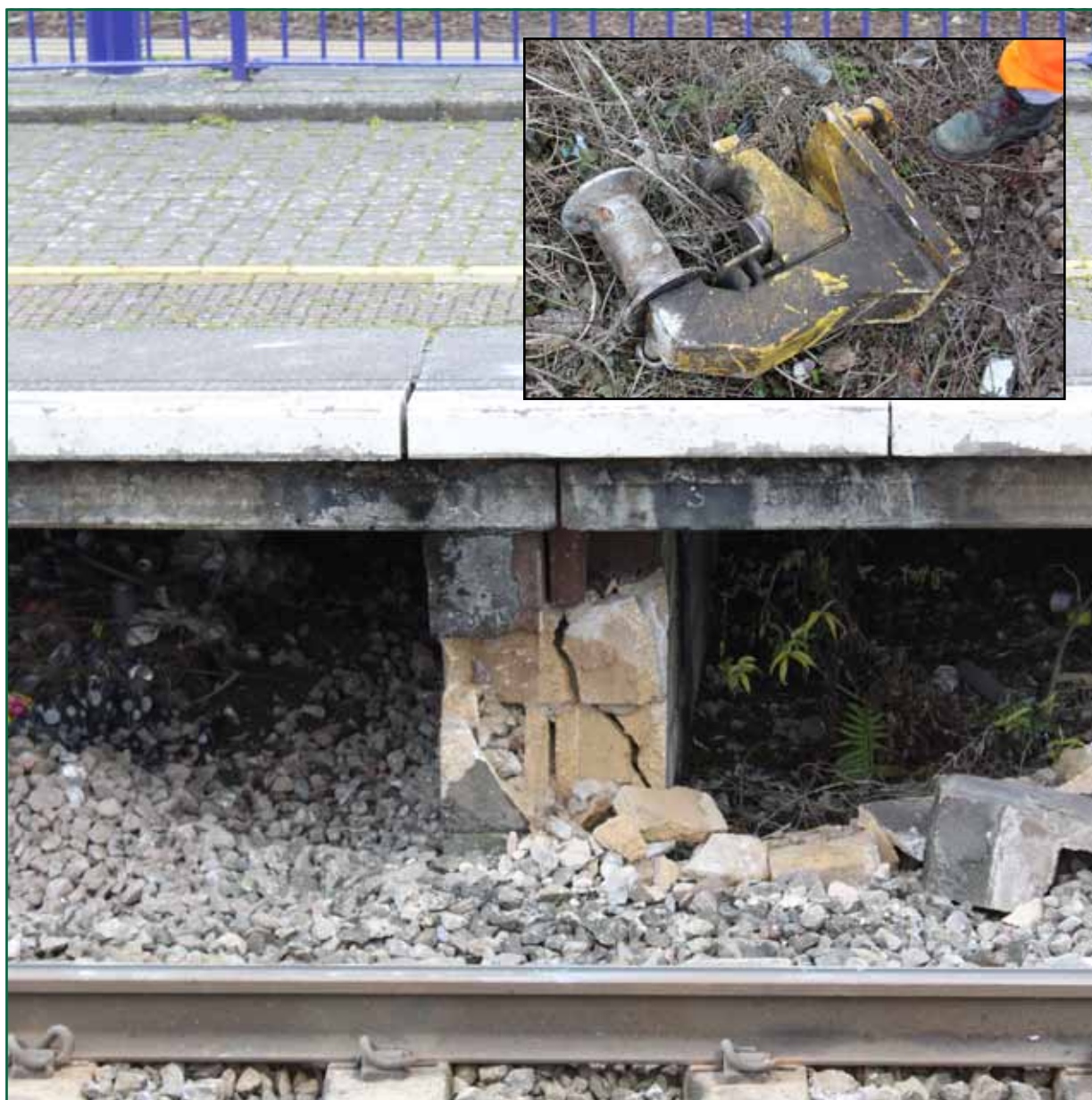
Figure 21: The damaged brick platform support at Thatcham station and the detached clamp (inset)
