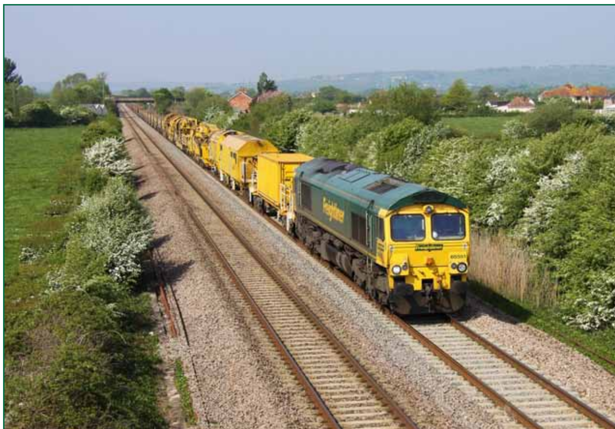
Figure 3: The track renewal train with support wagons (image courtesy of Stuart Graham of Stuart's Railway Photography)
