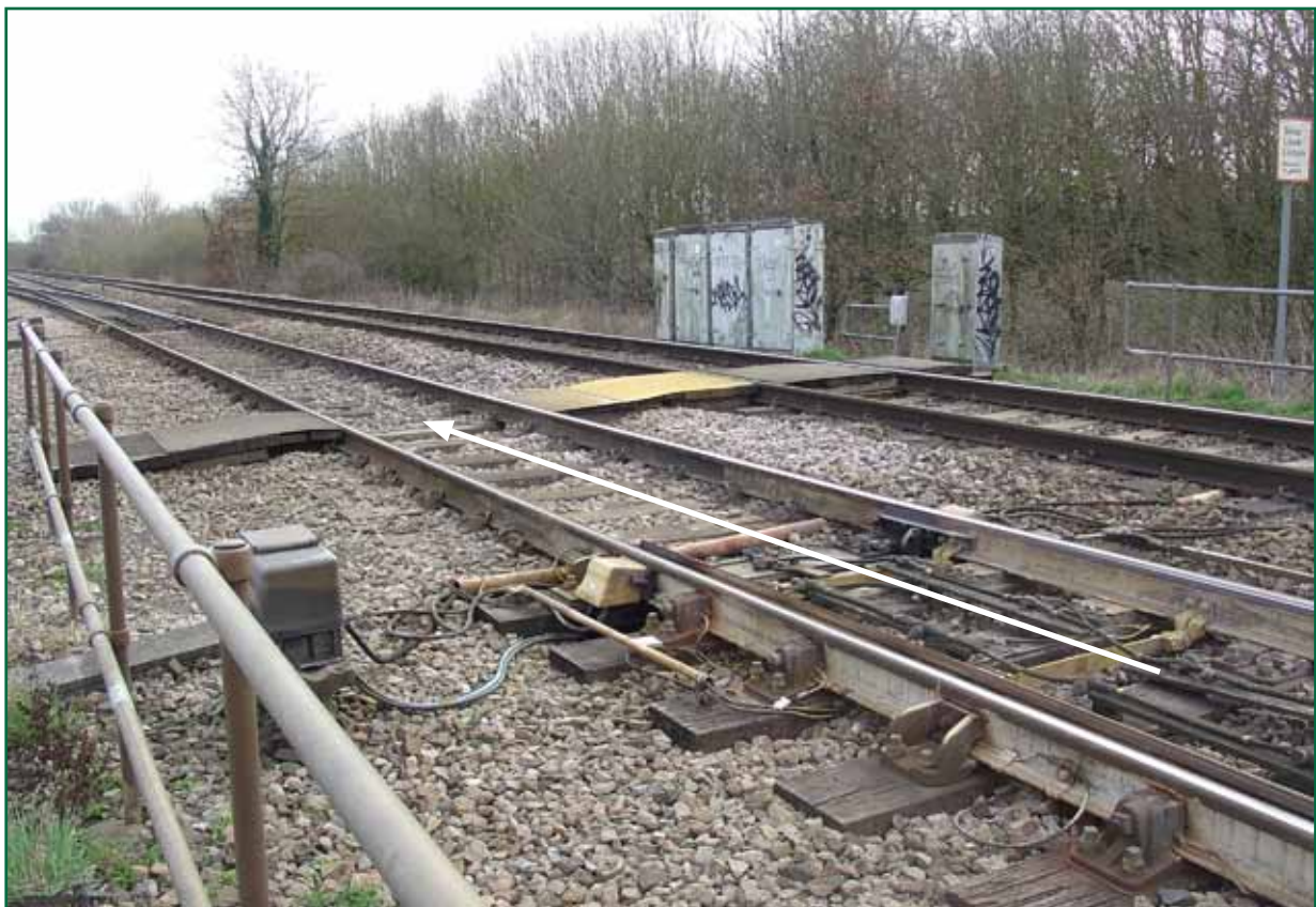
Figure 6: Blatchbridge Junction and the partially destroyed foot crossing (path of train 6Y33 indicated by white arrow)
