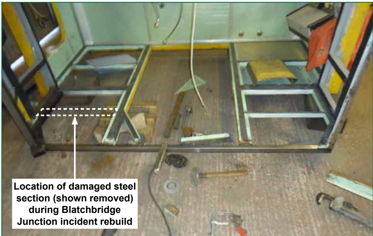
Figure 23: Damaged steel section removed for replacement during re-build of the P3 cab after the incident at Blatchbridge Junction. The front of the cab is lying face down in this image.
