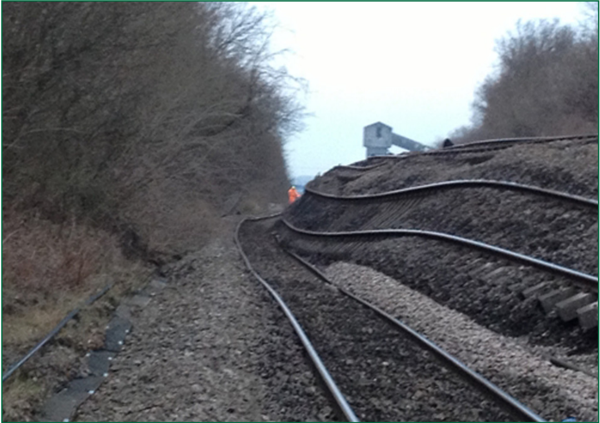
Figure 30: Hatfield Colliery: track deformation (image courtesy of Network Rail)
