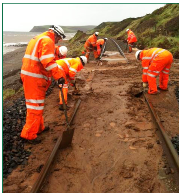
Figure 24: St Bees: October 2012 incident (image courtesy of Network Rail)
