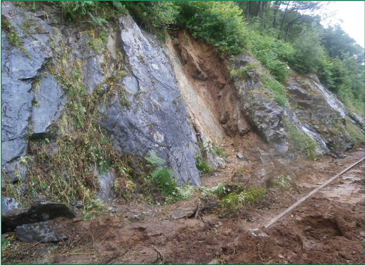
Figure 12: Falls of Cruachan: material washed from cutting face
