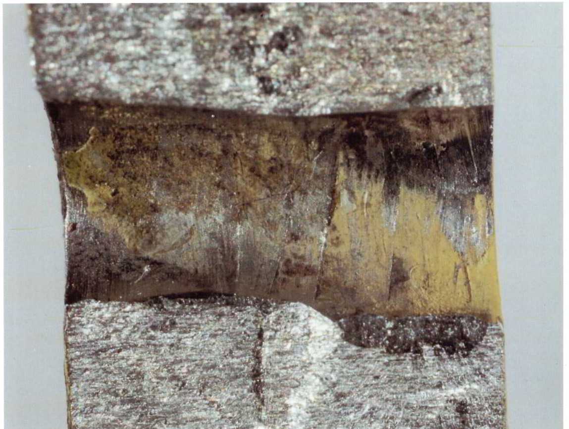
Photograph 2 Close up of damaged rivet hole (note scoring of hole surface and uneven shape)
