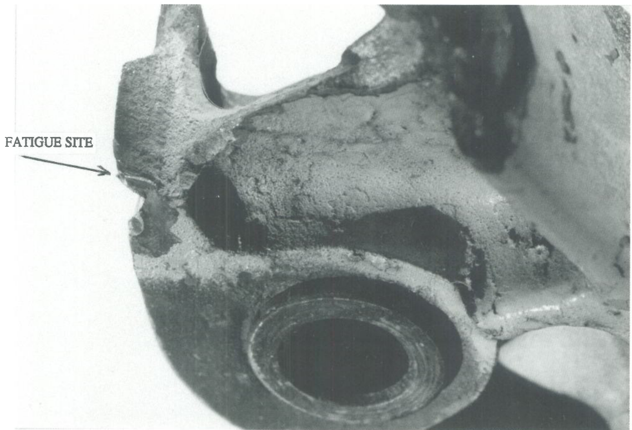
Fig 2 Area of Fatigue Damage
