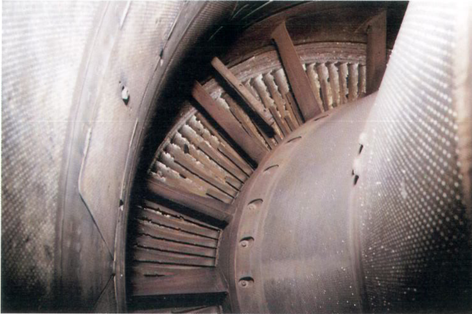
PHOTOGRAPH SHOWING DAMAGE TO L.P. TURBINE COMPONENTS.
