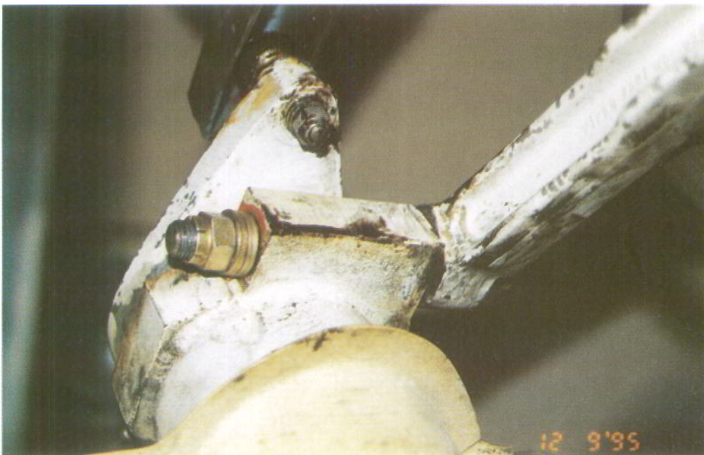
View of top of nose leg of G-BVEV, showing how upper drag link is attached to RHS of leg
