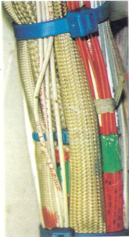
Wire damage at location A in figure B-2. Three wires affected in addition to scuffing of braided sheath.
