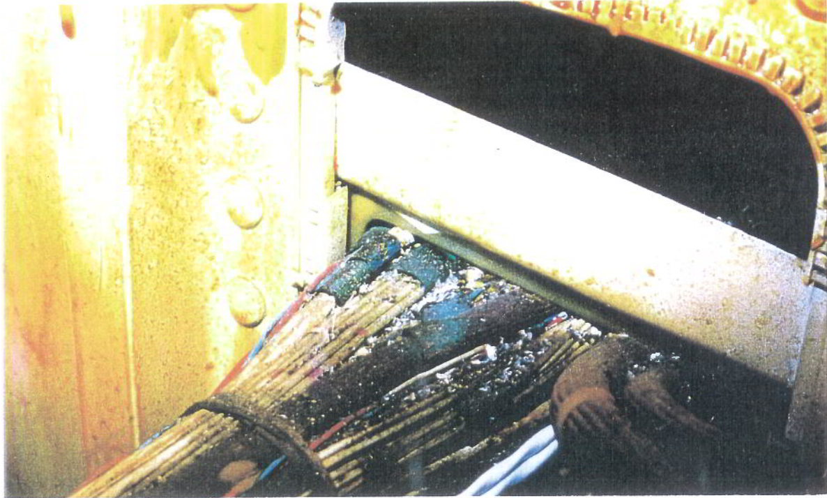
Contamination of wiring looms by drilling swarf, found in a retired B747, above, and an A300, below.
