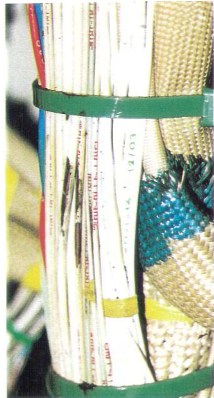
Abrasion of insulation topcoat at location B in figure B-2.
