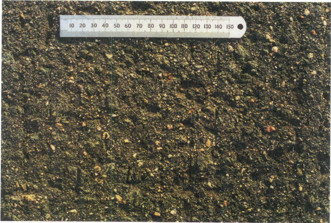
Figure 3 Close-up of old weathered runway surface at thresholds
