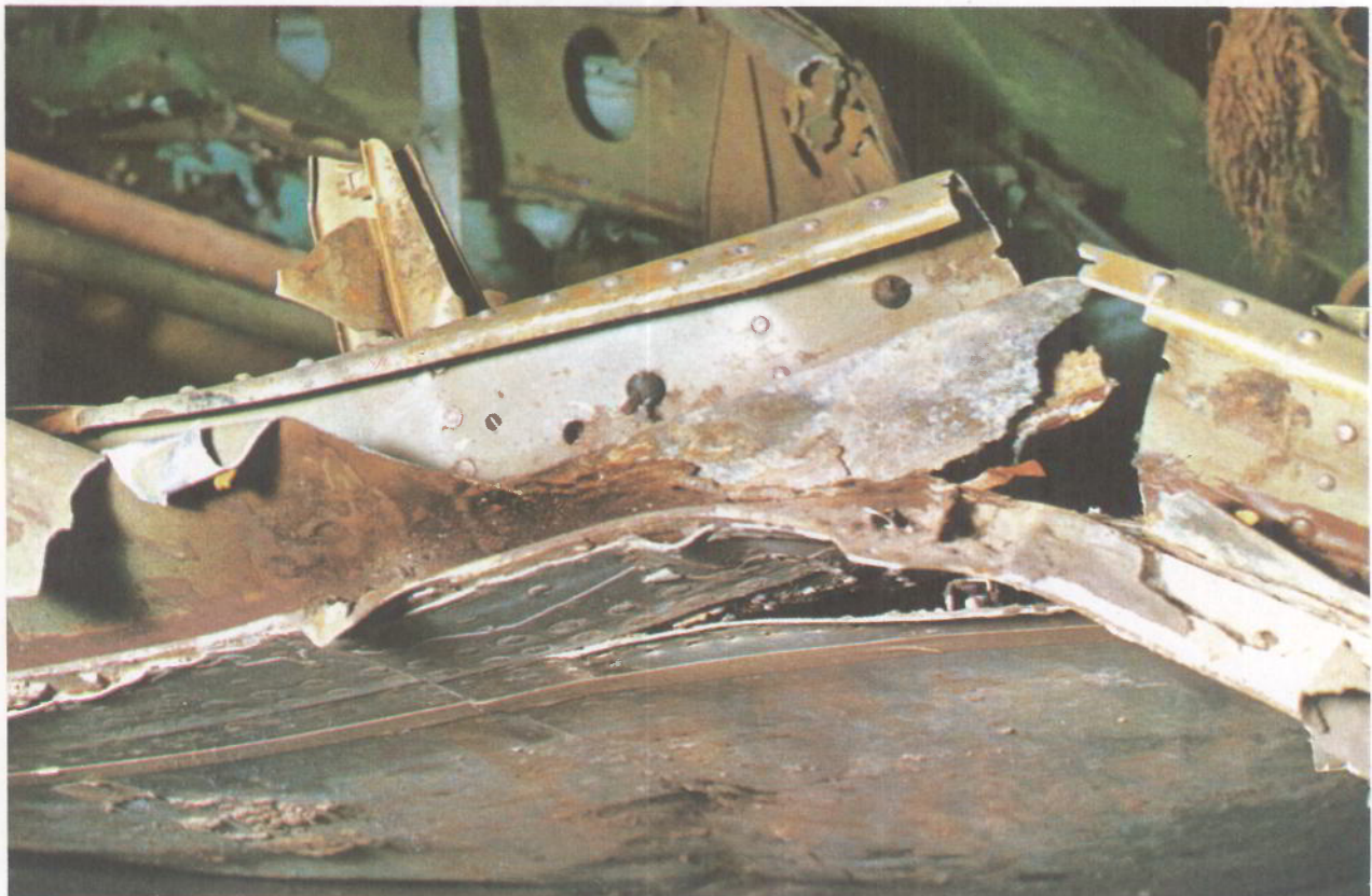
Figure n° 8: Lower portion of frame 1223 and rear pressure bulkhead, showing tar marks.
