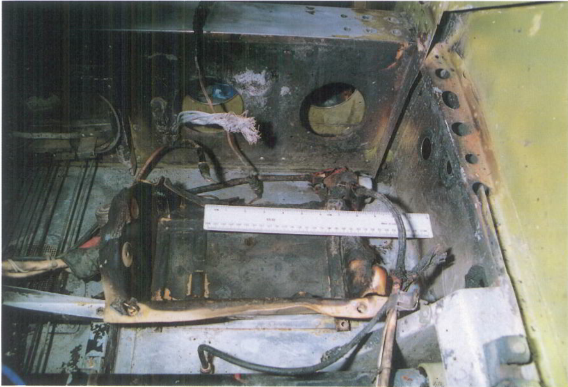
Figure 3 G-BNXT: Battery compartment after fire (Showing remains of bottom part of battery box and earth cable. Viewed looking forward from baggage door on starboard side of fuselage)
