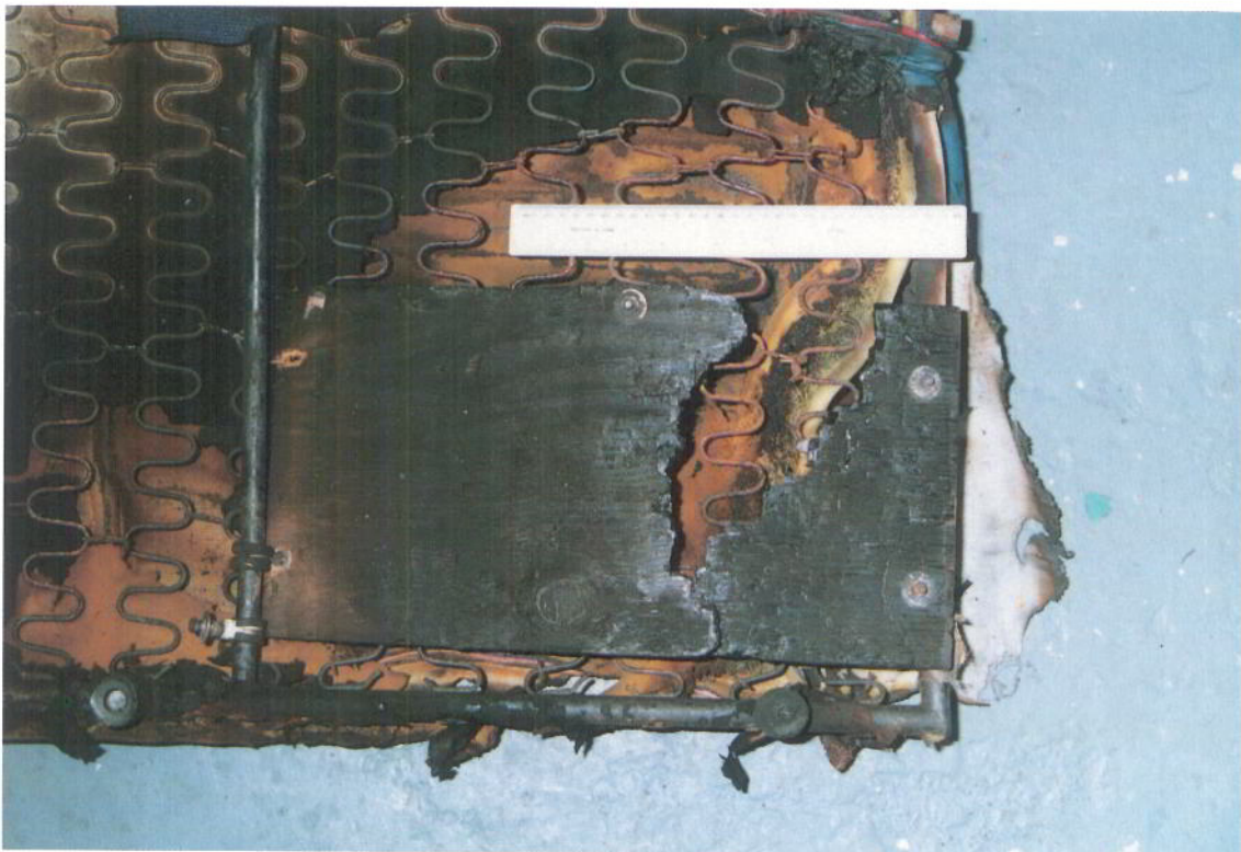
Figure 4 G-BNXT: Underside of rear starboard passenger seat Showing extensive fire damage including complete penetration of plywood board attached to underside of seat springs, to prevent springs contacting battery components.
